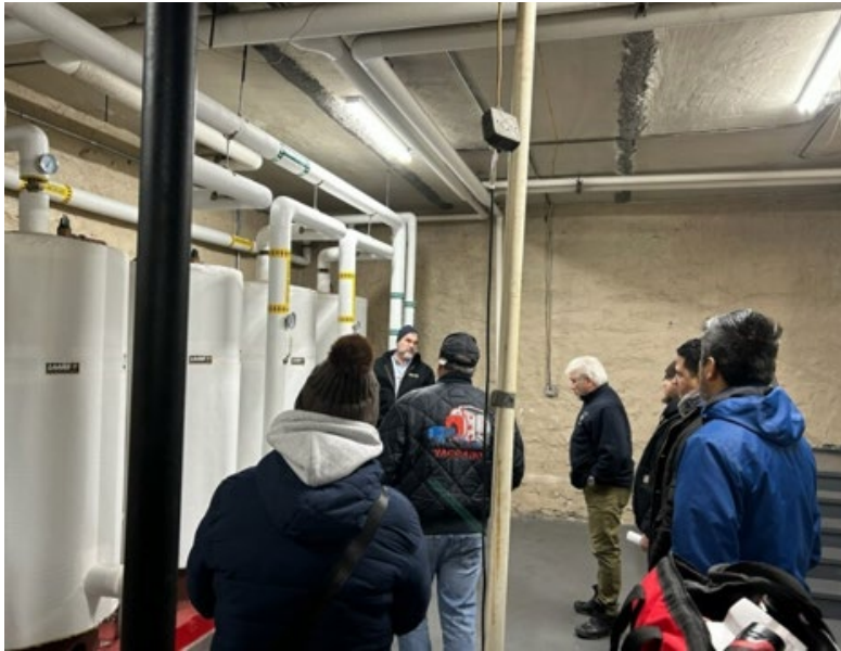
LAARS E-therm heat pump water heater training
